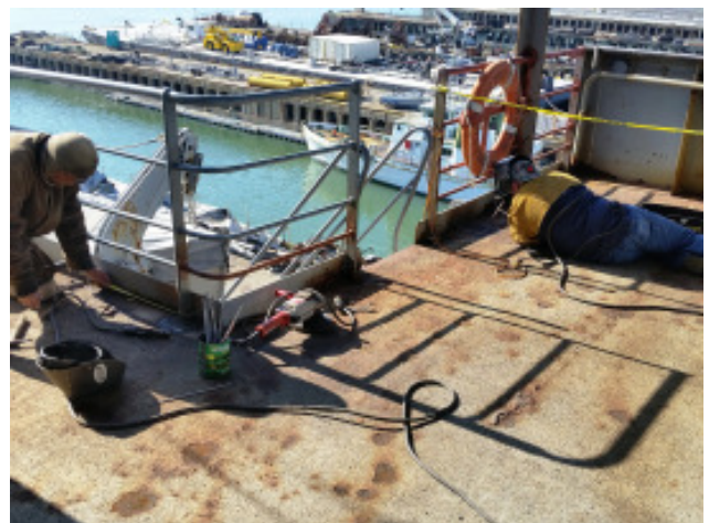
Lying down on the job! Red Oak Victory welders Mike Nagamoto (left), and Stanley Buck repair areas of the bridge deck that have rusted through. (Photo by Fred Klink)
