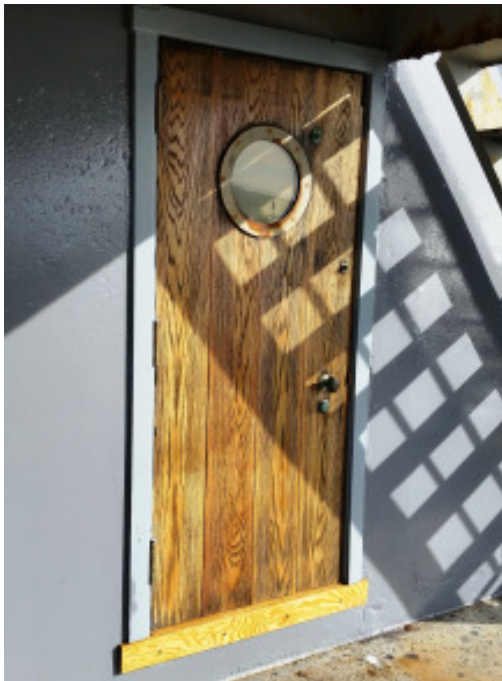
Port-side of the wheelhouse with refinished door, freshly painted bulkhead, and new threshold. (Photo by Fred Klink)
