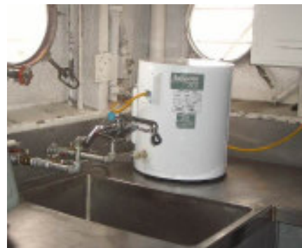
New water heater.
