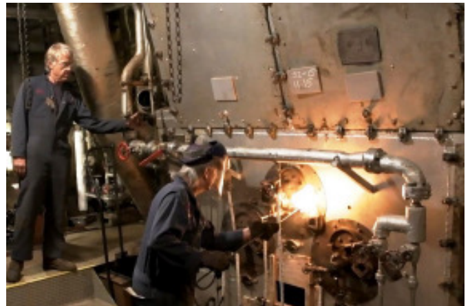
Greg Blasquez, Red Oak Victory Chief Engineer, lights off the middle burner of the starboard side boiler. (Photo by Dori Luzbetak)
